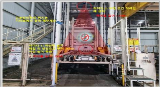
Example of field installation (Kia Motors Gwangju Autoland)
